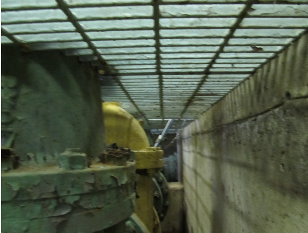
11) Sub grade piping with peeling and delamination to the underlying coats and to the substrate.
