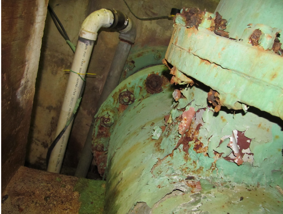
21) Nuts and bolts on the influent sub grade piping are in poor condition and actively corroding.
