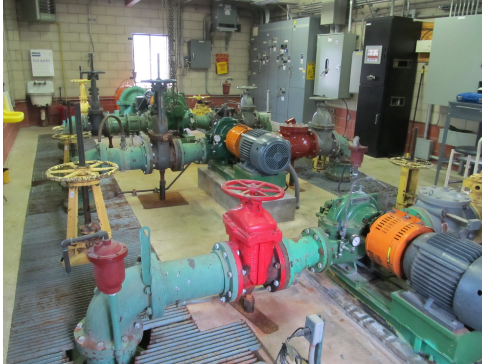
3) Piping is located above and below grade.
