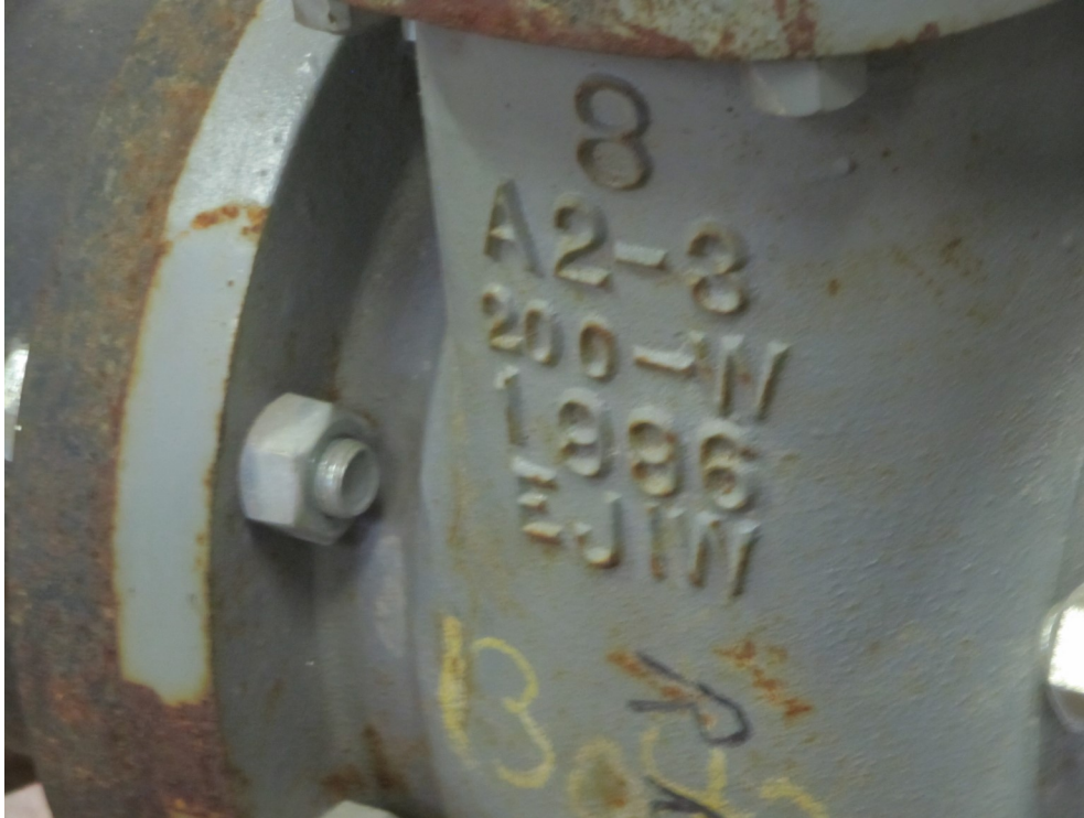
16) Piping, fittings, and pumps range from 1949 to 1996. Surface rusting is prevalent throughout.
