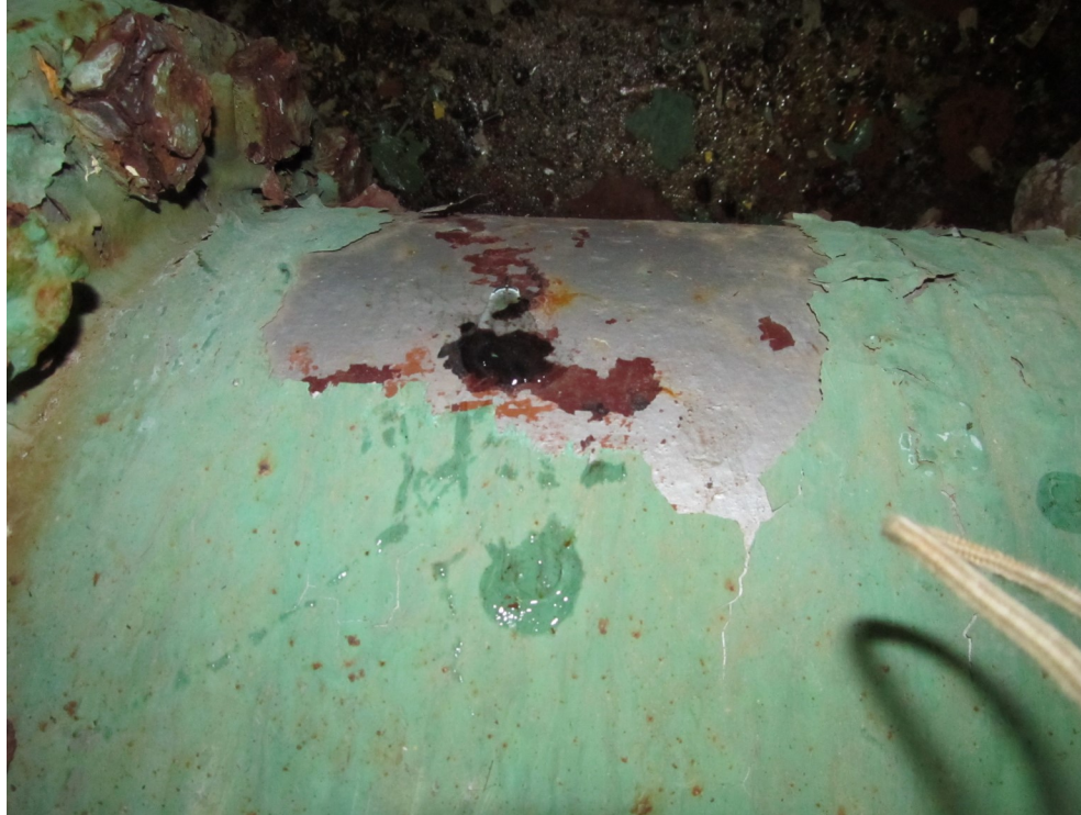
26) Lab samples taken indicate this is an alkyd system that is heavy metal bearing.
