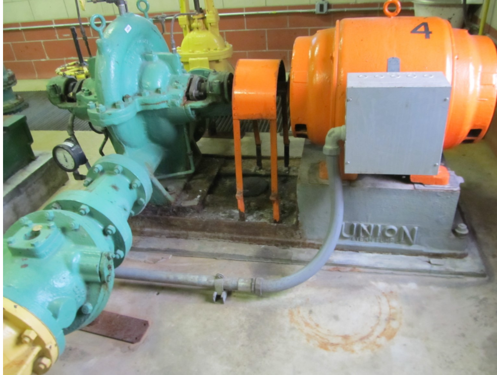
19) This pump appears to be from the original installation.
