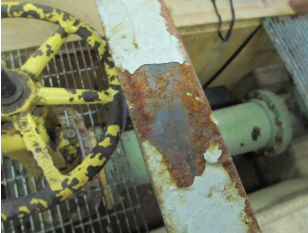
15) There is mill scale on the grating.
