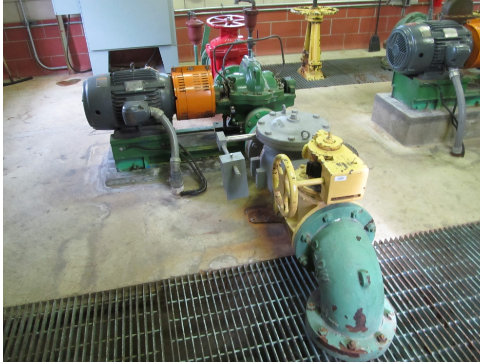
4) Various modes of coating failures were observed including abrasions, rust undercutting, and delamination to the substrate.
