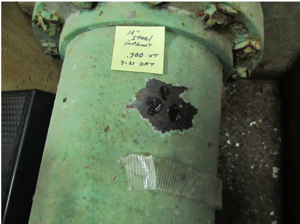
10) Dry film thickness, ultrasonic steel thickness, and adhesion testing was performed on the piping.
