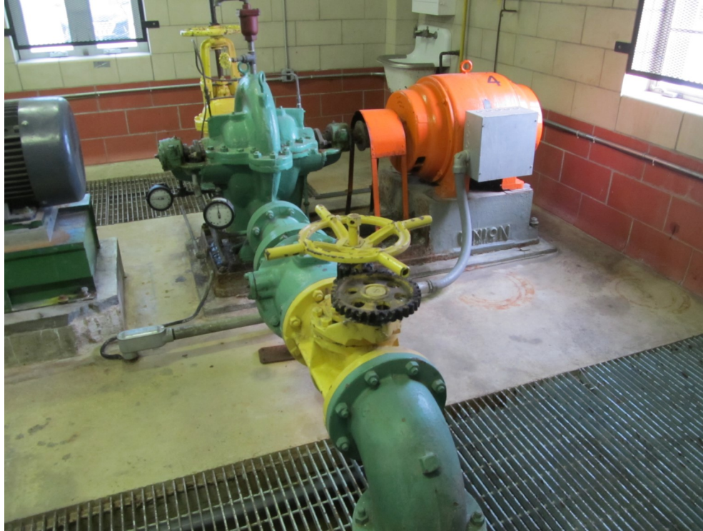
5) There are three pump stations with effluent piping.
