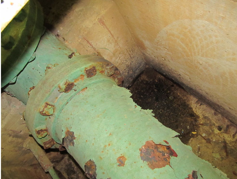
23) Corroding nuts, bolts, and coating failures on the piping. There is no significant steel loss on the piping exterior.
