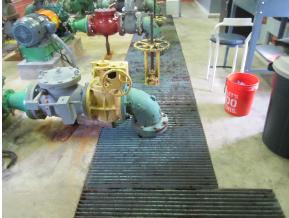
6) Valves and fittings been replaced and were left in primer. Many nuts and bolts have been replaced.
