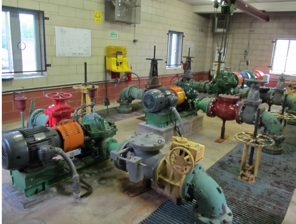
2) Booster Pump station with below grade influent and effluent. Three split case end suction horizontal booster pumps.
