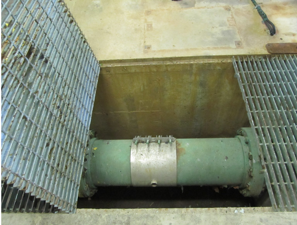
9) Effluent piping with tapping saddle, it is unknown if it is being utilized as a repair clamp.
