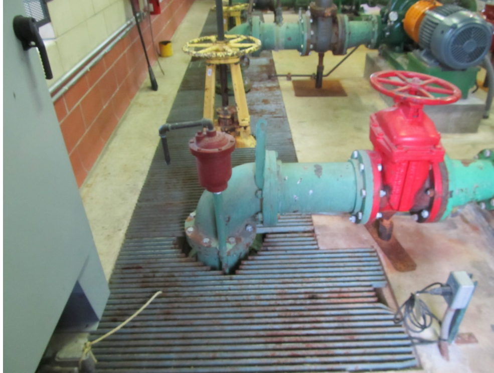
7) Influent piping is located under the removable grating.
