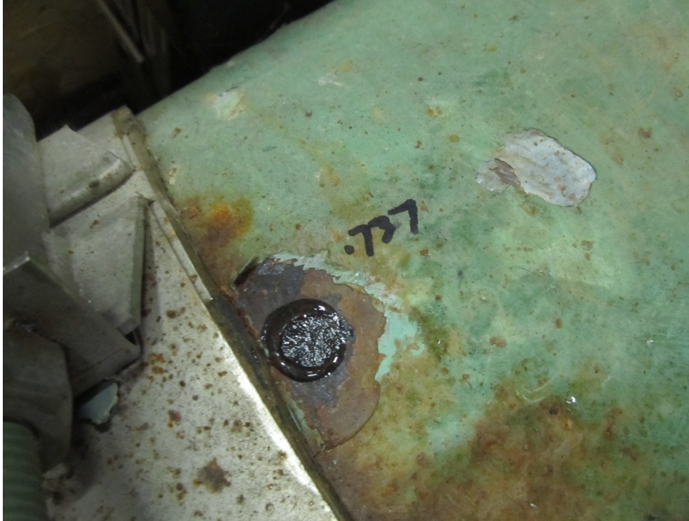
14) UT testing on adjacent surfaces to saddle indicate surfaces are 0.737 inch.
