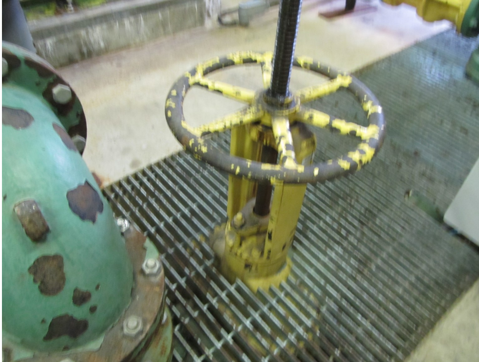
18) Spot coating failures to the substrate.
