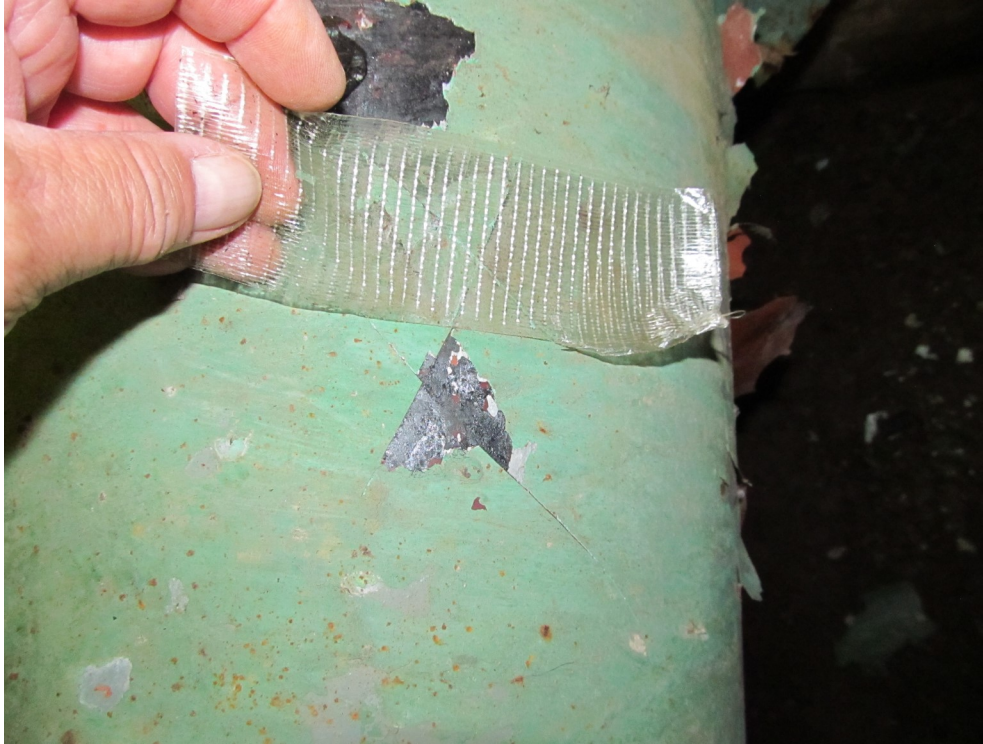
12) There is poor adhesion with coating failures to the substrate.
