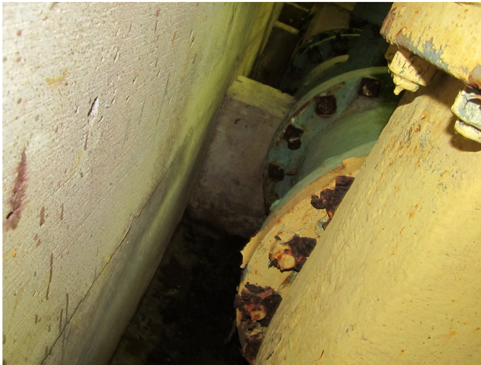
22) Bolt heads and nuts under grating are corroding.
