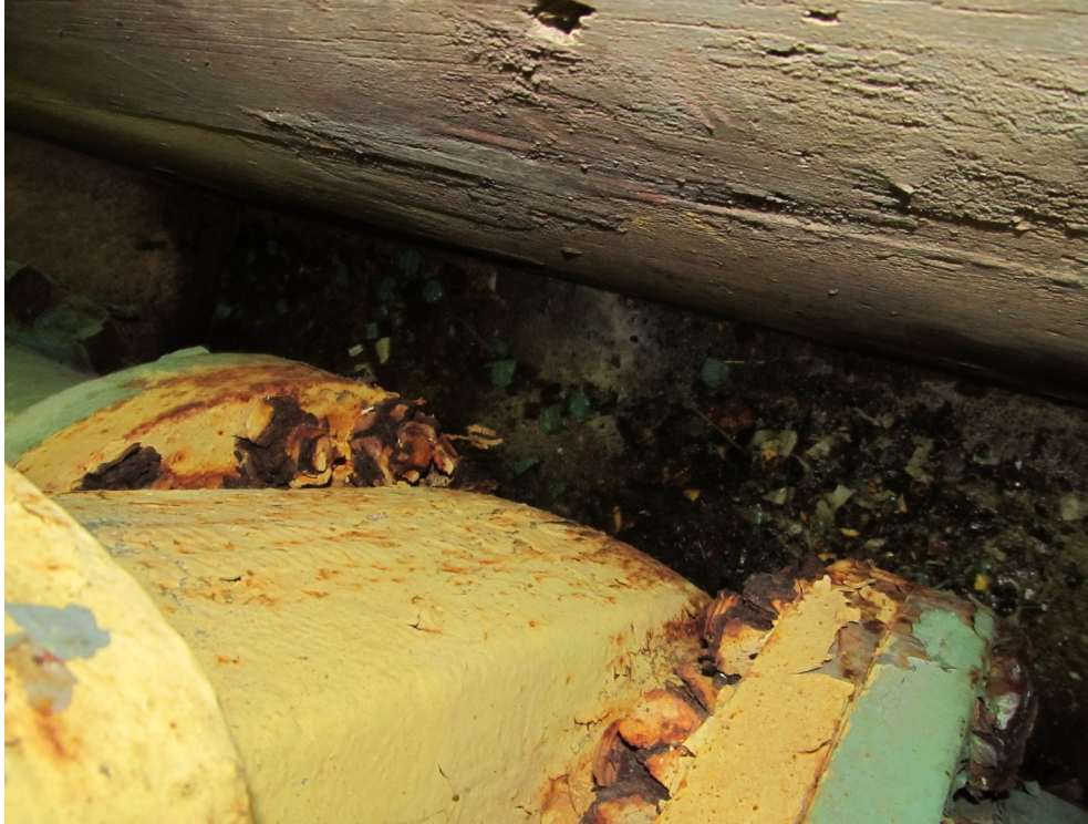
27) Difficult to access, nuts and bolts that are severely corroded with steel loss.
