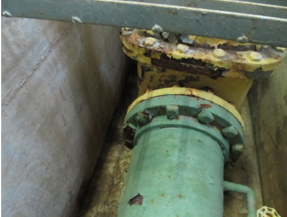
24) Coating failures to the substrate on valves, fittings, and pipe.
