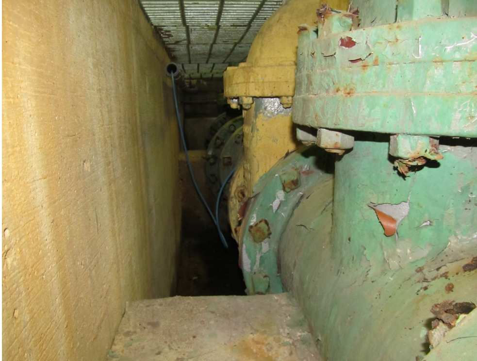
13) There is limited access to sides and bottom of the piping. The nuts and bolts are corroding.
