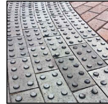
TRUNCATED DOME BRICK PAVERS (OAKLAND ST. & FARMINGTON ST. PLAZAS ON WEST SIDE OF INTERSECTION)
