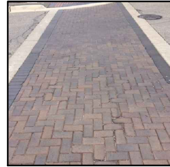
HERRINGBONE BRICK PAVER CROSSWALK (OAKLAND ST. & FARMINGTON ST. CROSSWALK, ON WEST SIDE)
