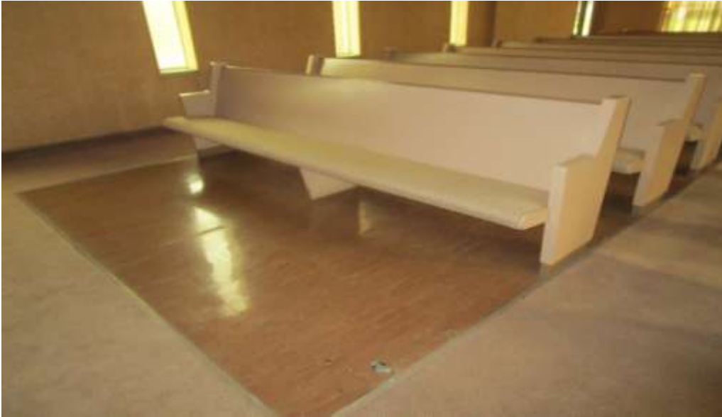
Picture of asbestos containing floor tile in church under pews/carpet.
