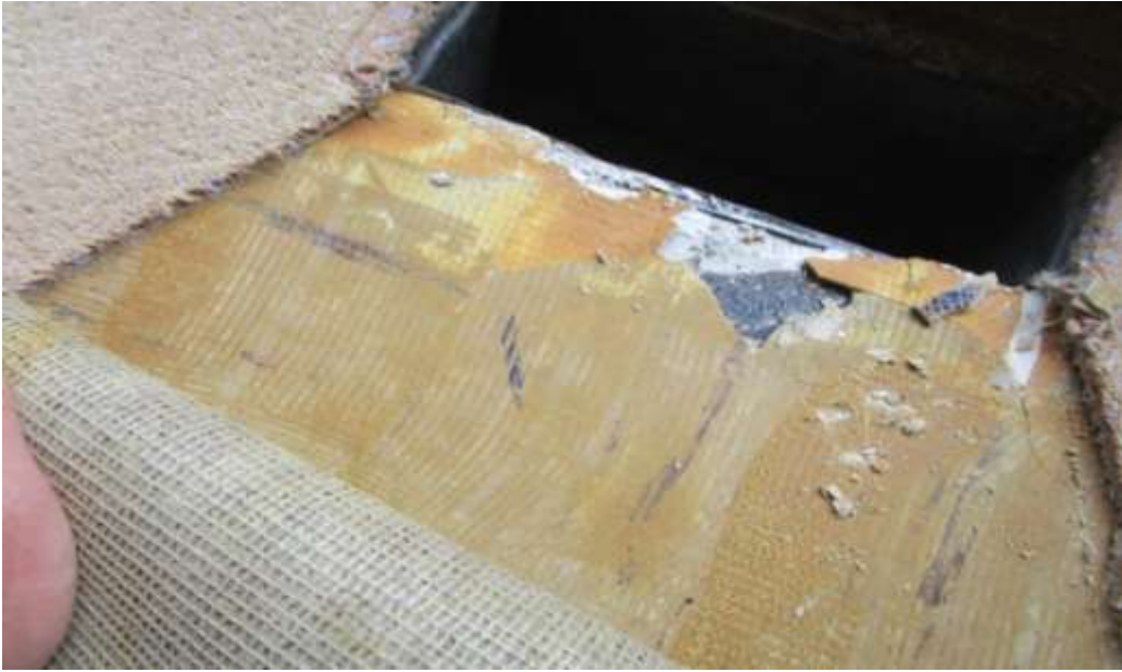
Asbestos containing floor tile under carpet northeast Corner on main floor and throughout.
