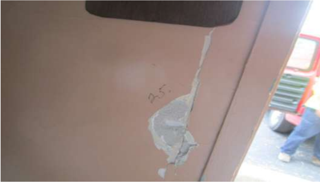
Asbestos containing plaster in stairway from basement South entrance.
