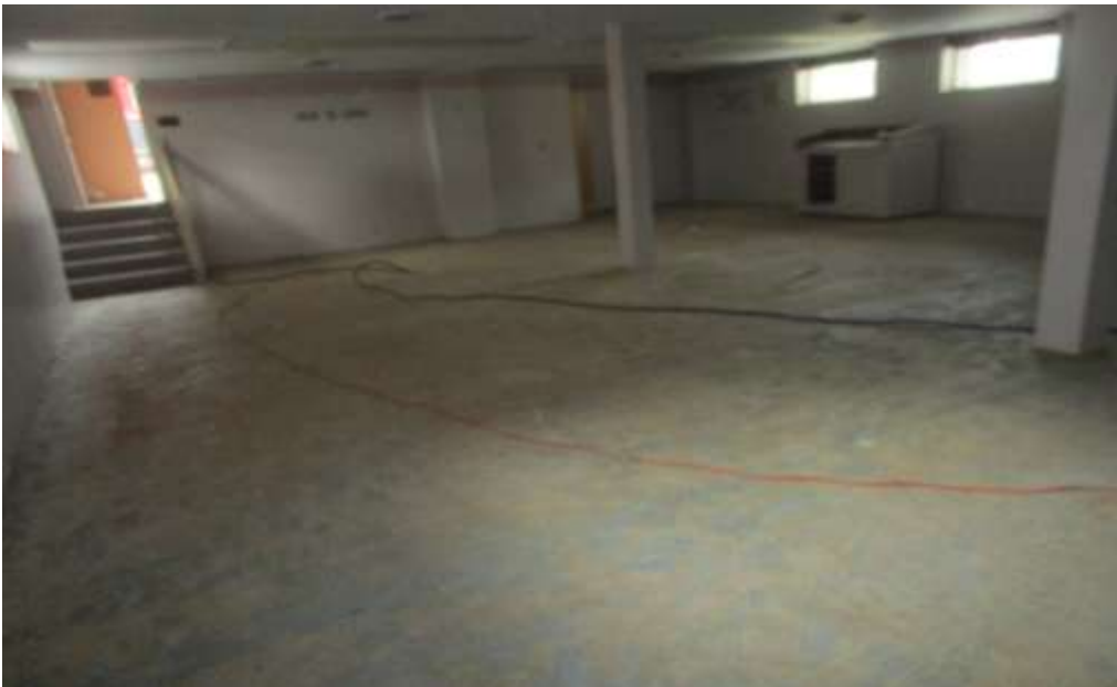
Asbestos containing floor tile in basement.
