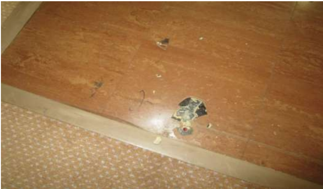
Asbestos containing floor tile (2 layers) in church under pews and carpet throughout.
